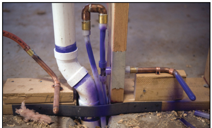
Pipes and fittings that are part of the reclaimed waste water system are spray painted purple in accordance with the CID modification of Appendix J 5 of the 2003 UPC [Section 1617.0 of the 2006 UPC].
