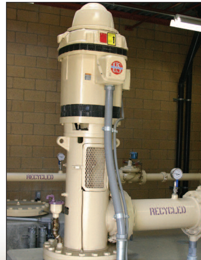
This 200 horsepower pump in a Chino Hills, California booster station is capable of pumping 1440 gallons of recycled water per minute. The station houses three 200 horsepower pumps and one 25 horsepower pump; up to 2 million gallons pass through the station each day.
